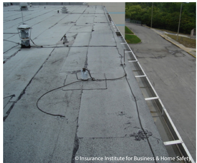
An example of a modified bitumen roof cover with aluminum gutters free of debris (including the granules from the roof cover system).
